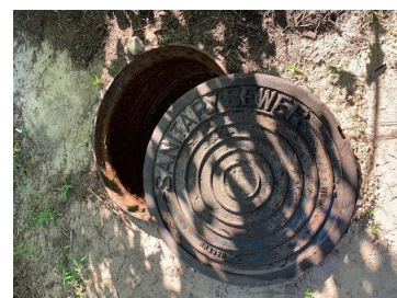
Grease Traps Did you know SJRA inspects hundreds of grease traps (aka interceptors) around The Woodlands, Texas? A grease trap
