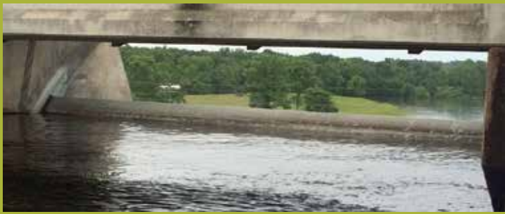
Figure 4. This photo shows the top of one of the main spillway gates at the Lake Conroe dam. At normal pool level of 201' MSL, there is approximately 18 inches of "freeboard" above the water line.
