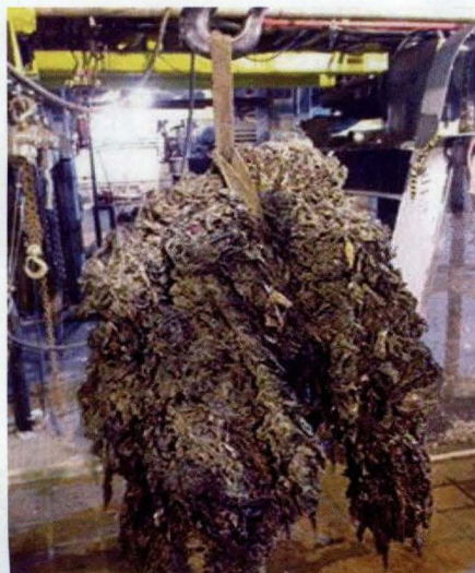
A disgusting tangle of wipes trapped in sewer equipment.
