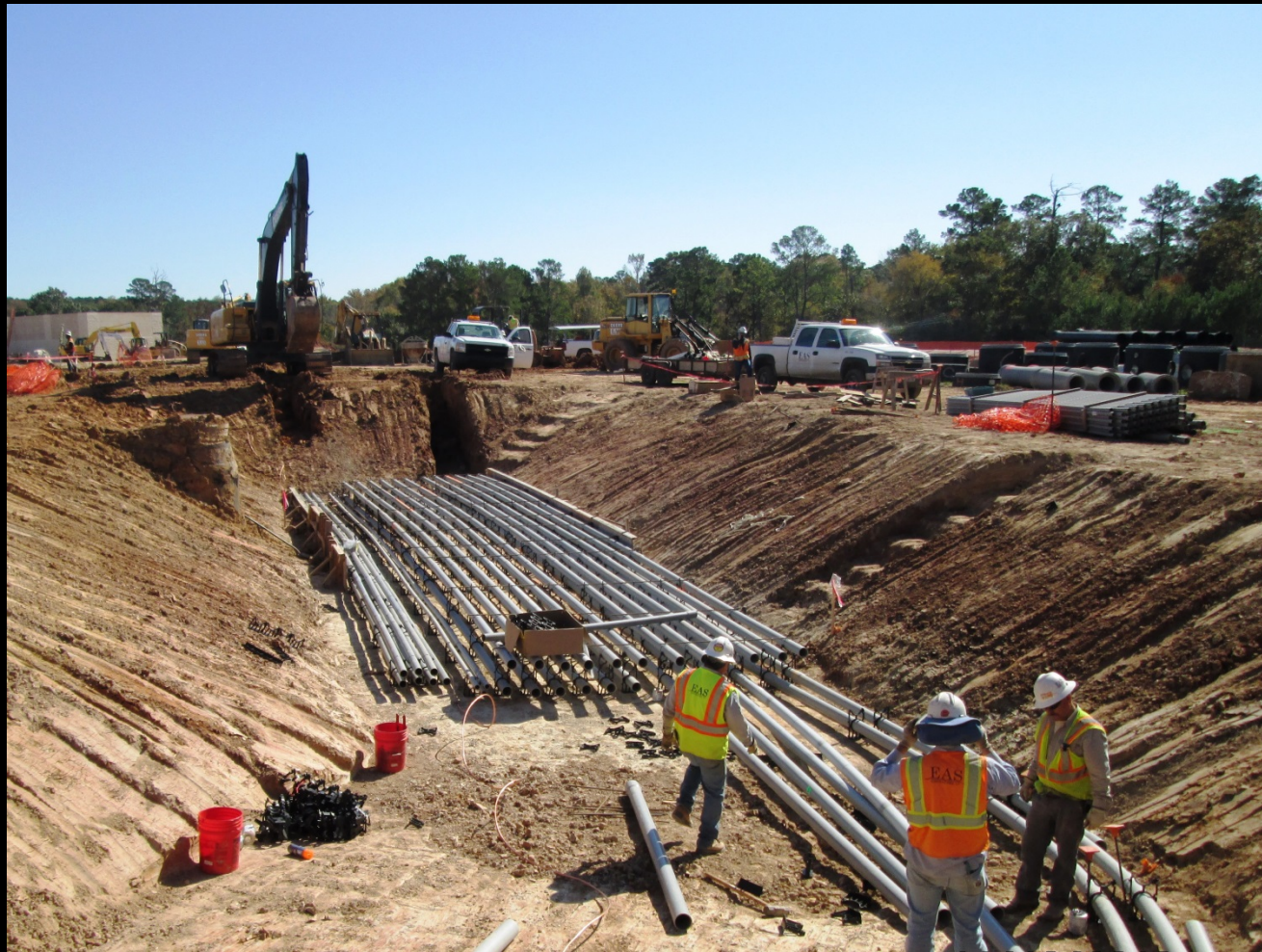
Electrical duct bank from Electrical Building to the High Service Pump Station
