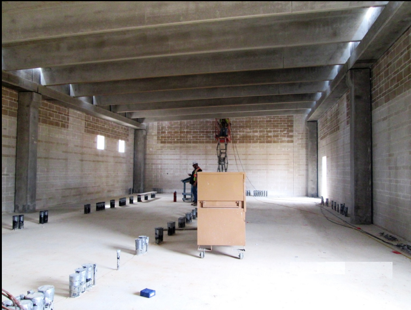
Interior view of Electrical Building
